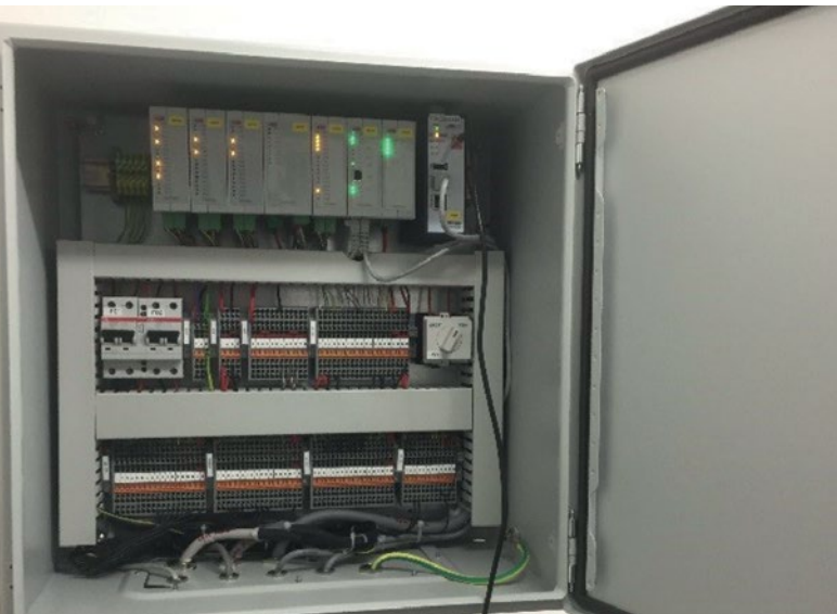
01 Ready to install wall-mounted cabinet
