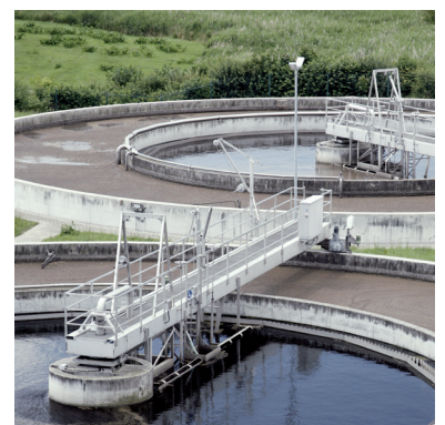
Water treatment plants
