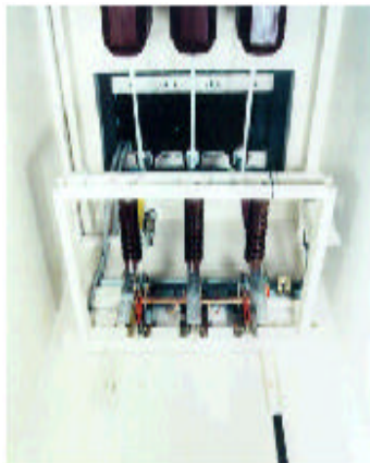
Earthing switch EK6 with motorised mechanism.
