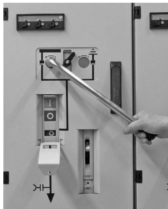
Fig. 4.1.2.1.2.2: Operation of the three position disconnecter (in this case disconnecter operation) with manual mechanism 1
