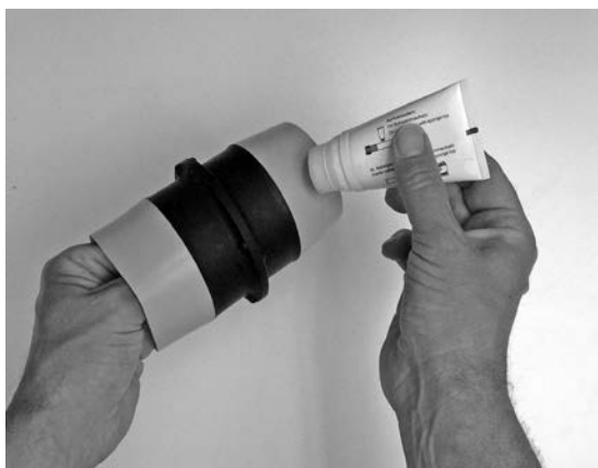
Fig. 2.1.3.1: Greasing the light, outer areas of the silicone insulating part on the busbar connection
