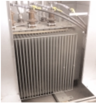
The oil collection pit protects the environment.
