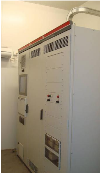
Fig. 6: SVC control room (MACH 2 and OWS)
