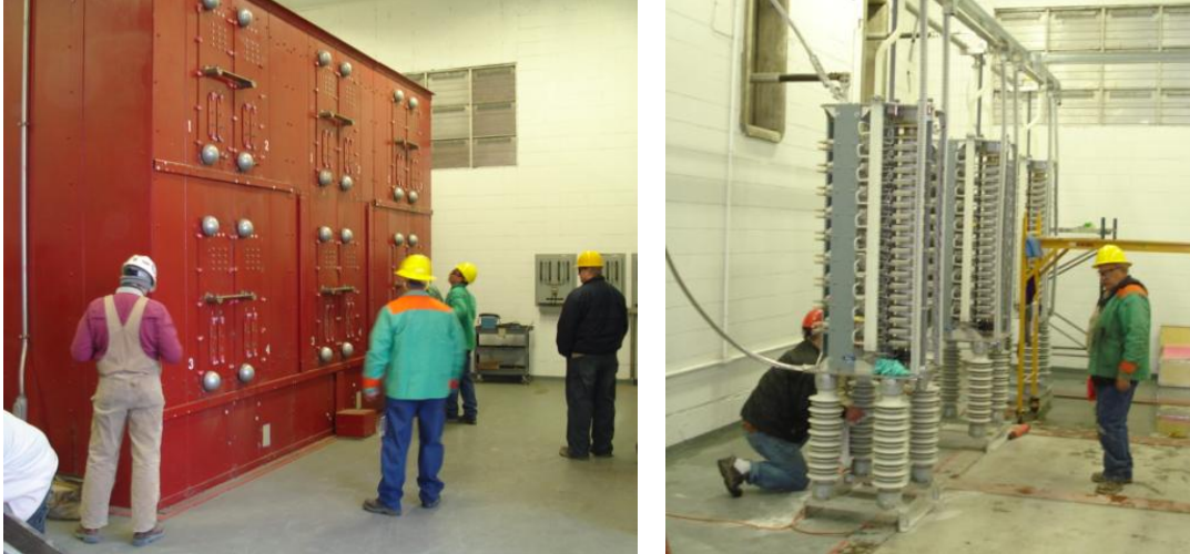
Fig. 10: (Left): Old GE thyristor valves from 1980. (Right): New ABB thyristor valves being installed next to the base of the old valves.
