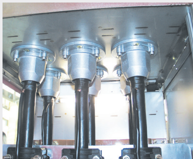
Cable termination compartment with inner cone connectors
