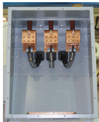
Main terminal box
