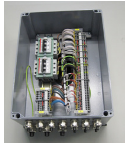
Auxiliary terminal box
