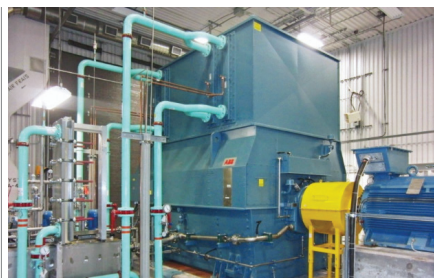
Above: Figure 1. ABB synchronous condenser
