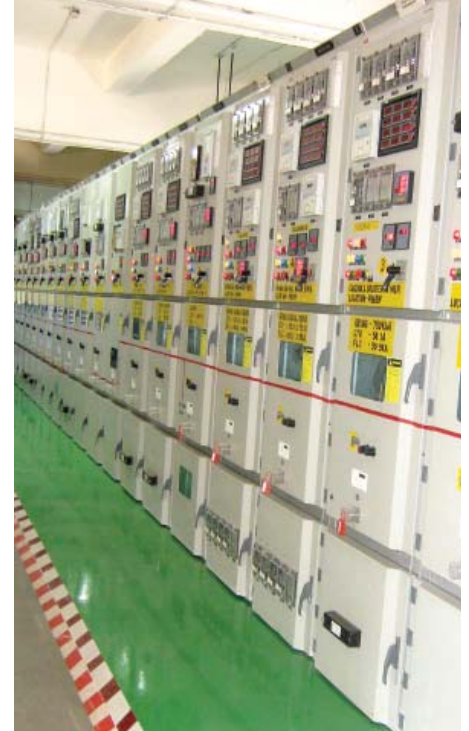
ABB installations at the plant
