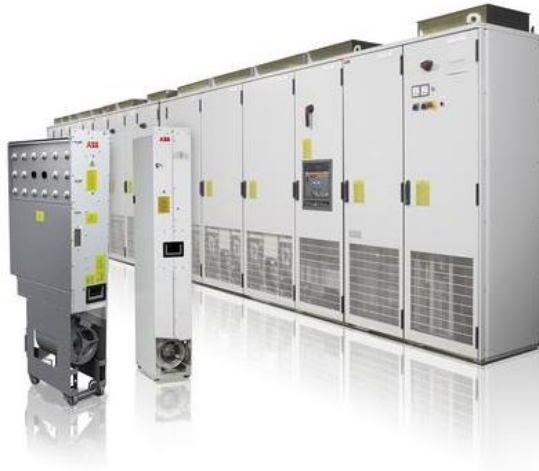
Figure 2. Air cooled Drive cabinet and Module
