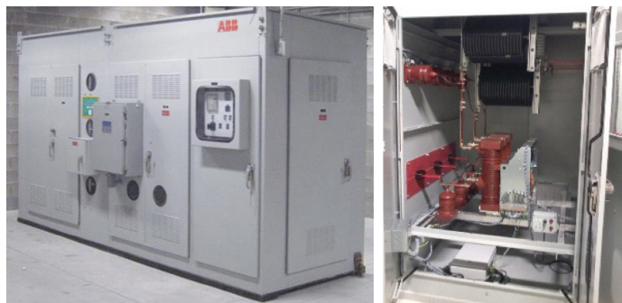
Figure 3 - 10 MVAR capacitor bank with DS1 inside.
