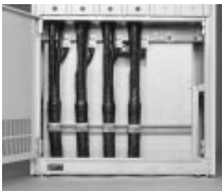
The supply cubicle has plenty of space for incoming cables.
