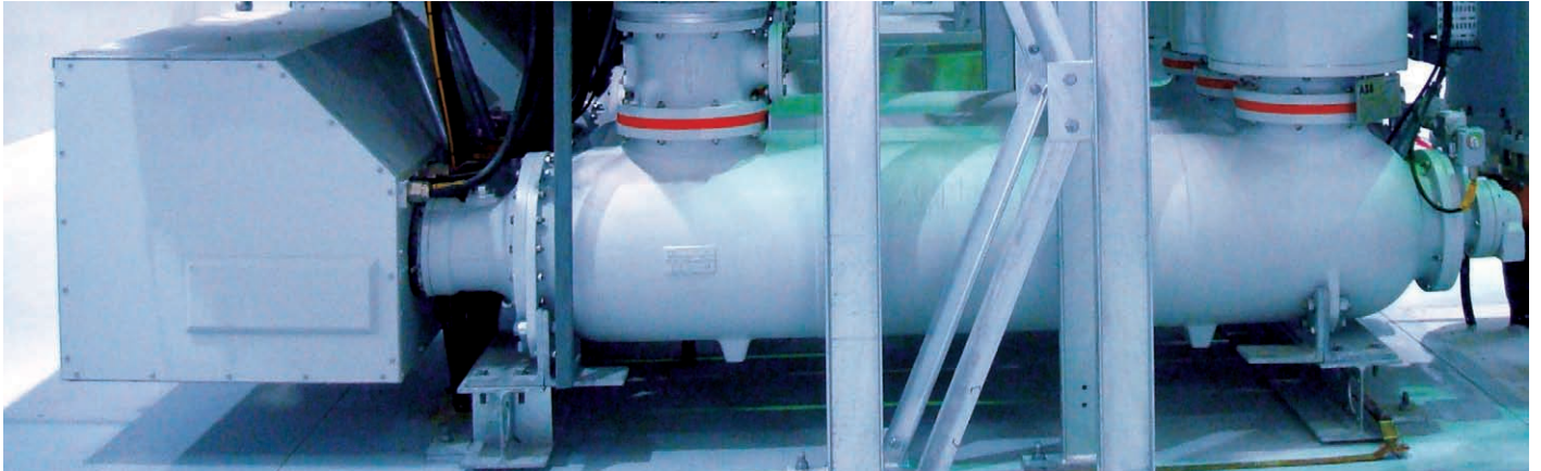
Circuit-breaker with operating mechanism
