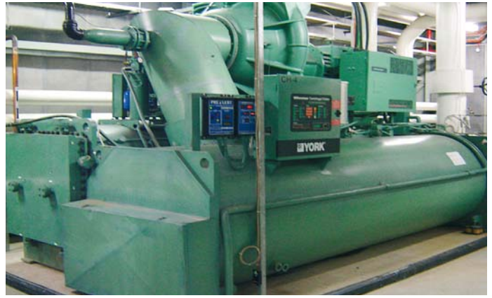
Throttling valves on the water-cooled chillers have been replaced with variable speed drives.
