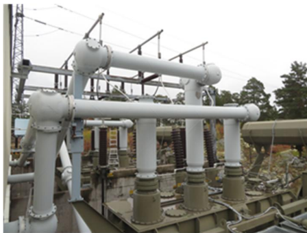
Figure 3 Gotland 2, Svenska Kraftnät, transformer to valve connection
