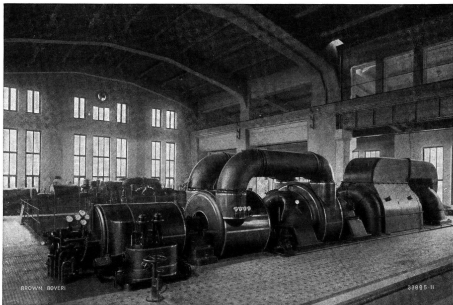
Fig. 8. — Power house of the Caroline Pit. The Brown Boveri turbo-set in foreground (see Fig. 7). Valve housing separate. U-shaped connection pipes between valve housing and nozzle boxes.
