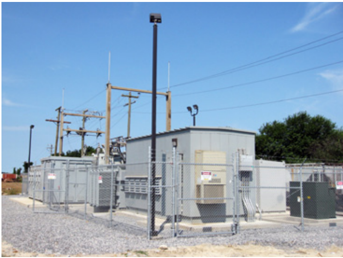
An ABB STATCOM installation for a car crusher facility in Virginia.
