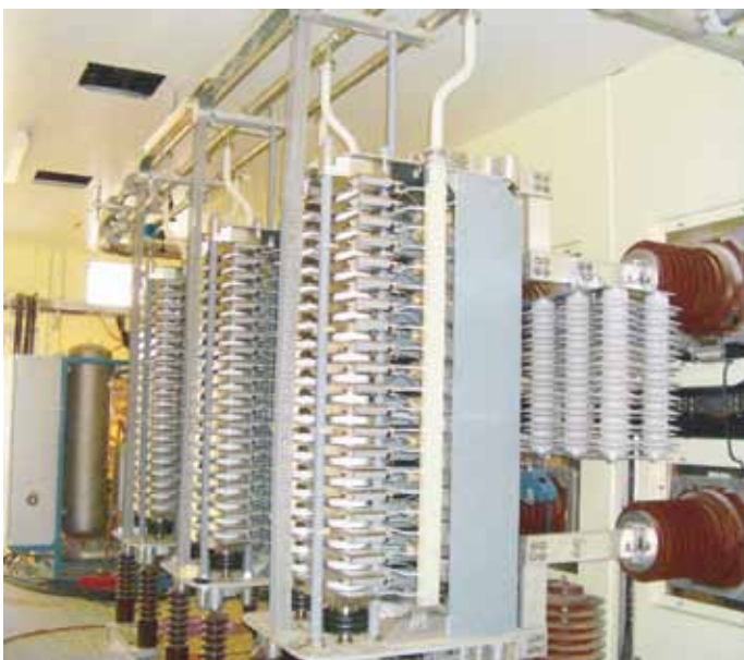
TSC valve and cooling equipment
