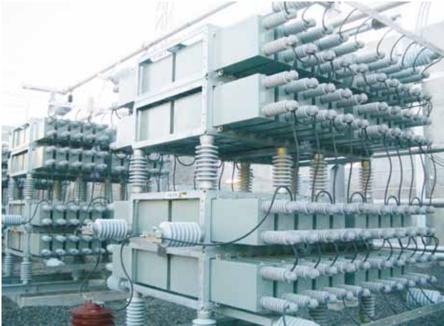
TSC capacitor bank
