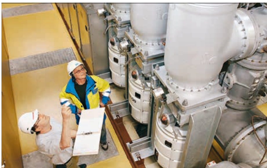
1 La Foretaille GIS substation in Switzerland. The older-generation circuit breaker type SN was replaced by an ELK SP2-1 with AHMA drive.
