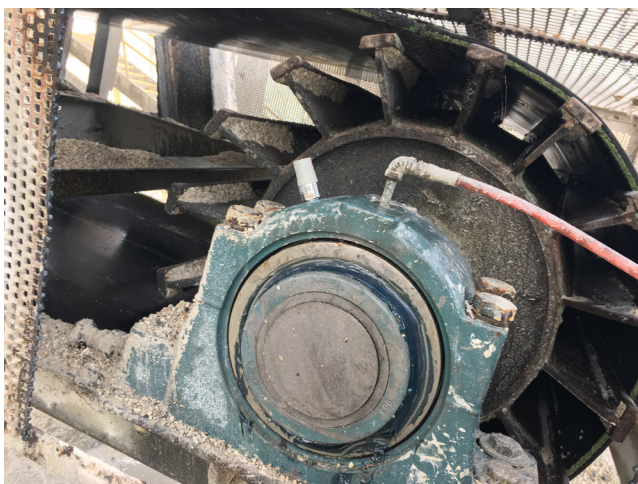
Figure 2. Smart sensors (shown here as the white cylinder on the bearing) allow equipment to be monitored in locations which may be difficult or dangerous to reach.
