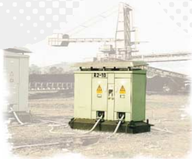
Stope switchgear unit in open-cast brown-coal mining
