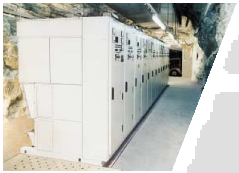
Gas-insulated switchgear, type ZV2 in salt mine
