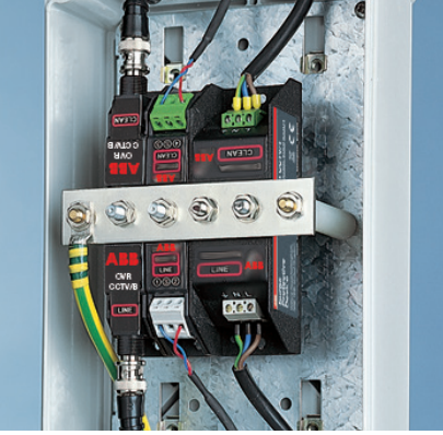
Figure 5: Installation of OVR 240-16A next to Video and Telemetry SPDs assembled on a CME kit.
