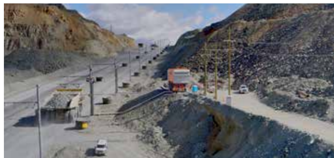
ABB eMine trolley system, with overhead catenary system and DC substation shown at Copper Mountain Mine. Image courtesy of Copper Mountain Mining
