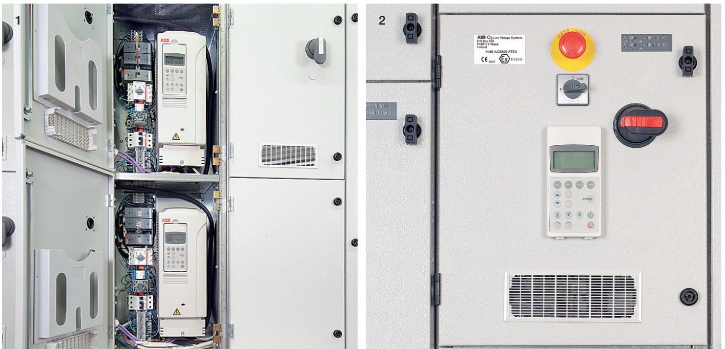
1 Switchgear mounted industrial drives | 2 ATEX certified ACS800 drives
