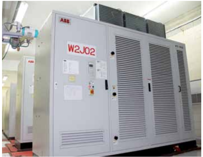
Air-cooled ACS 5000 variable speed drives controlling the flow rate of the preheater ID fans
