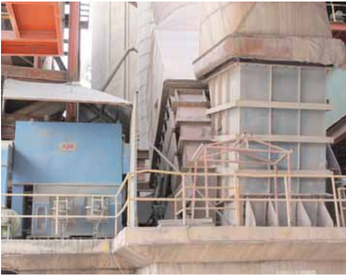
Motor and preheater ID fan at Siam City Cement's Saraburi cement plant in Thailand
