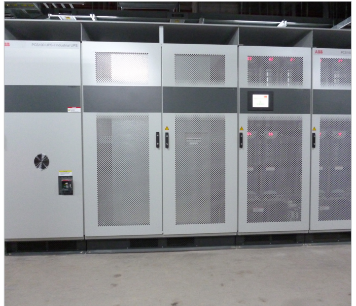
ABB's PCS100 Industrial UPS that has been installed for phase one in Samsung's Suzhou facility to protect against voltage sags
