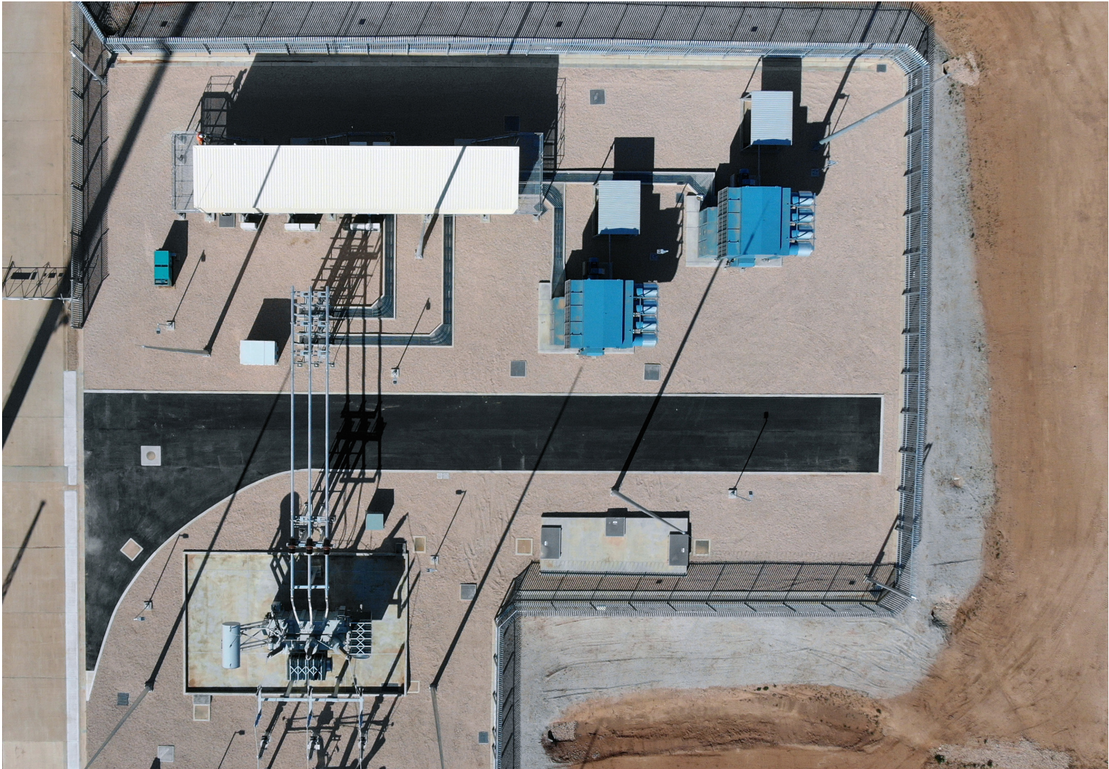
Darlington Point Solar Farm Project
