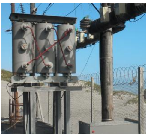
Fig. 3: Polemount dry-type transformer installed at KIPTS test station in South Africa. The Atlantic Ocean is seen in the background.
