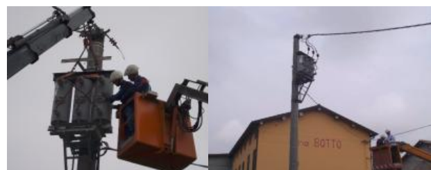
Fig. 8: Dry-type polemount transformer installed in the region of Brescia, Italy
