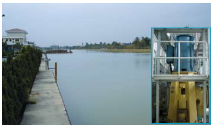
Raw water intake canal and vertical motor and pump at MWA's Mahasawat plant
