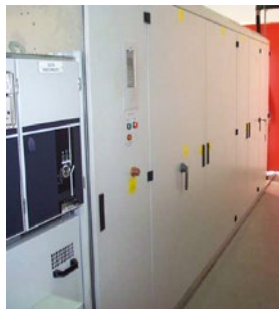
View of motor driven by ACS 1000; ACS1000 in converter building; Converter building and three-winding input isolation transformer.
