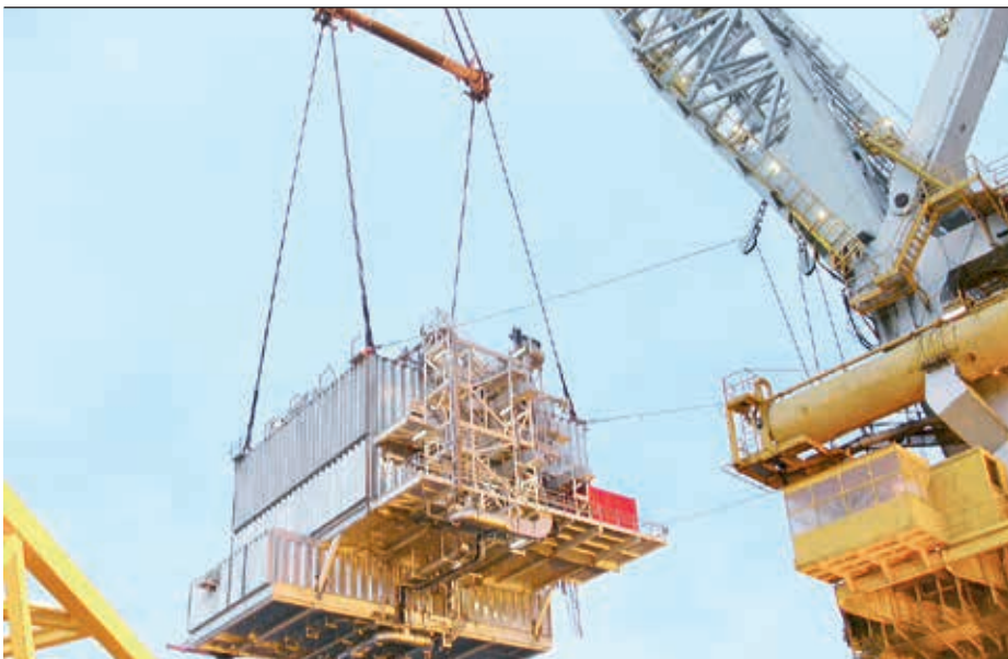
11 Lifting an HVDC Light offshore module into position on a North Sea oil platform.
