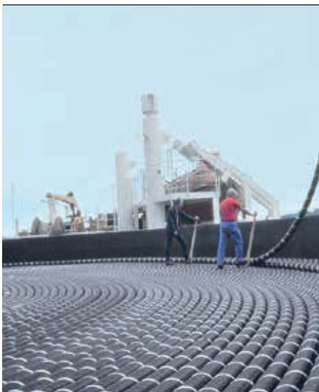
10 Cable of the Fenno Scan HVDC link being loaded onto a ship. This link was completed in 1989.
