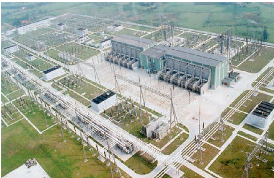
9 The Jingzhou station of the Three Gorges Guangdong HVDC link
