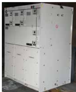
From IAC-test with arc suppressor
