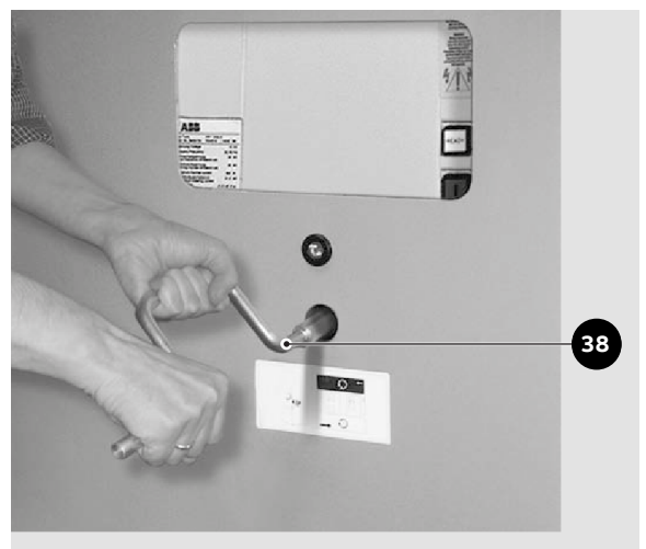
Figure 9/20: Moving the circuit breaker on a withdrawable part between the test/disconnected position and the service position; clockwise up to the stop for the service position and anticlockwise for the test/disconnected position. Example of a panel. 38 Hand crank
