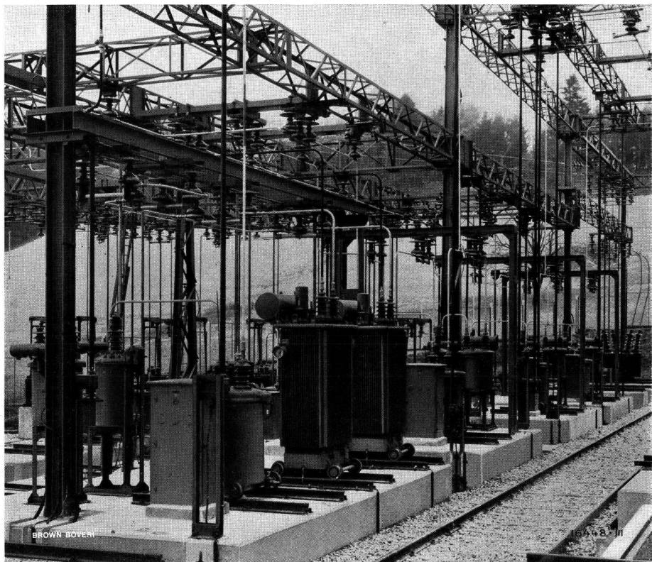
Fig. 10. — View of part of the Puidoux plant with station transformers.
