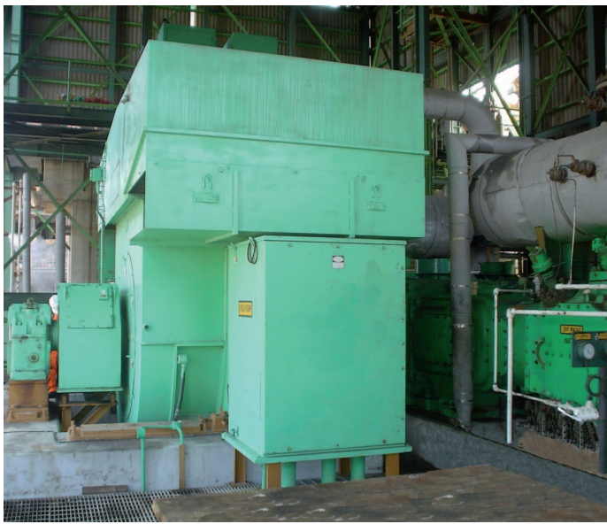
View of motor and compressor (5500 kW)
