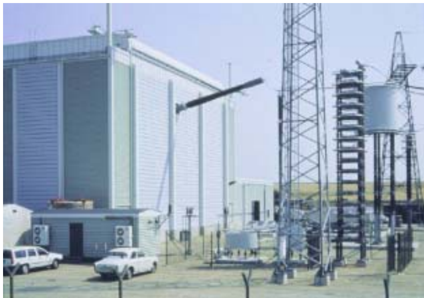
Figure 10 Active filter cubicle and dc filter in front of valve hall at Kruseberg, Baltic Cable
