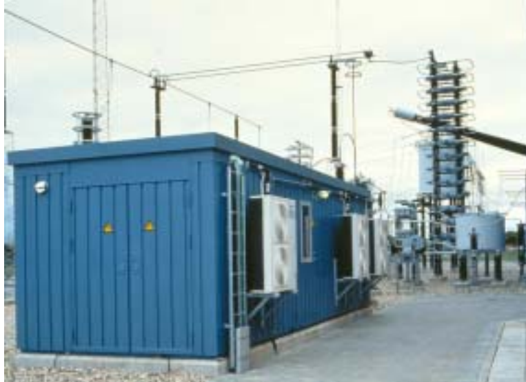
Figure 7 Active filter cubicle in front of dc filter at Tjele, Skagerrak 3
