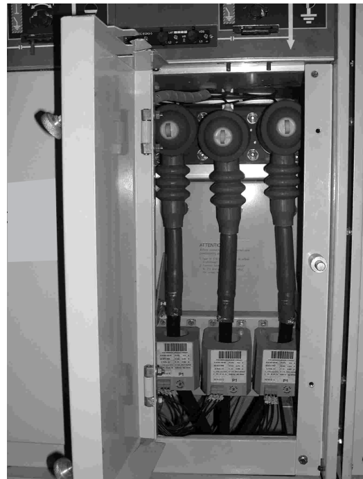
3 core cable termination with CT mounted.
