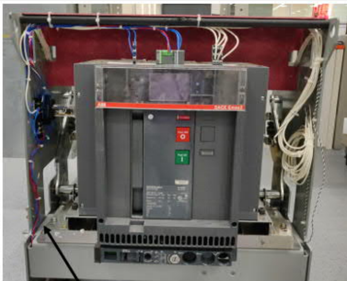
Wiring of WP 4000A Breaker with Fan Control Unit
