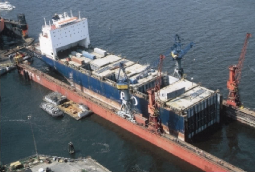
Sea-Land Pride (formerly Galveston Bay) in Dock 10 after the forebody had been cut away. The midbody is being prepared for removal. 2
