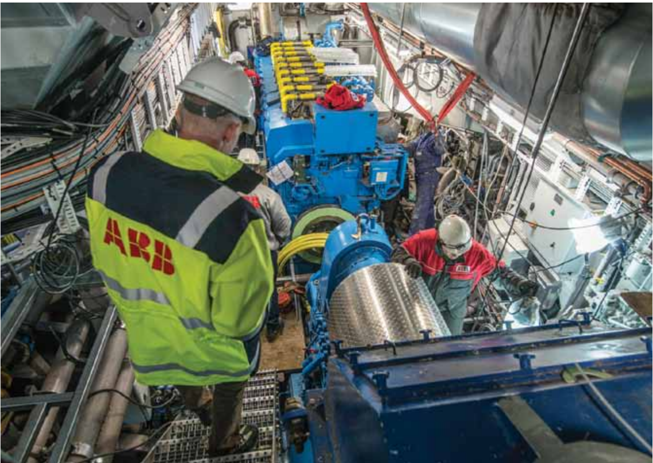
Marine Harvest feeder engine room
