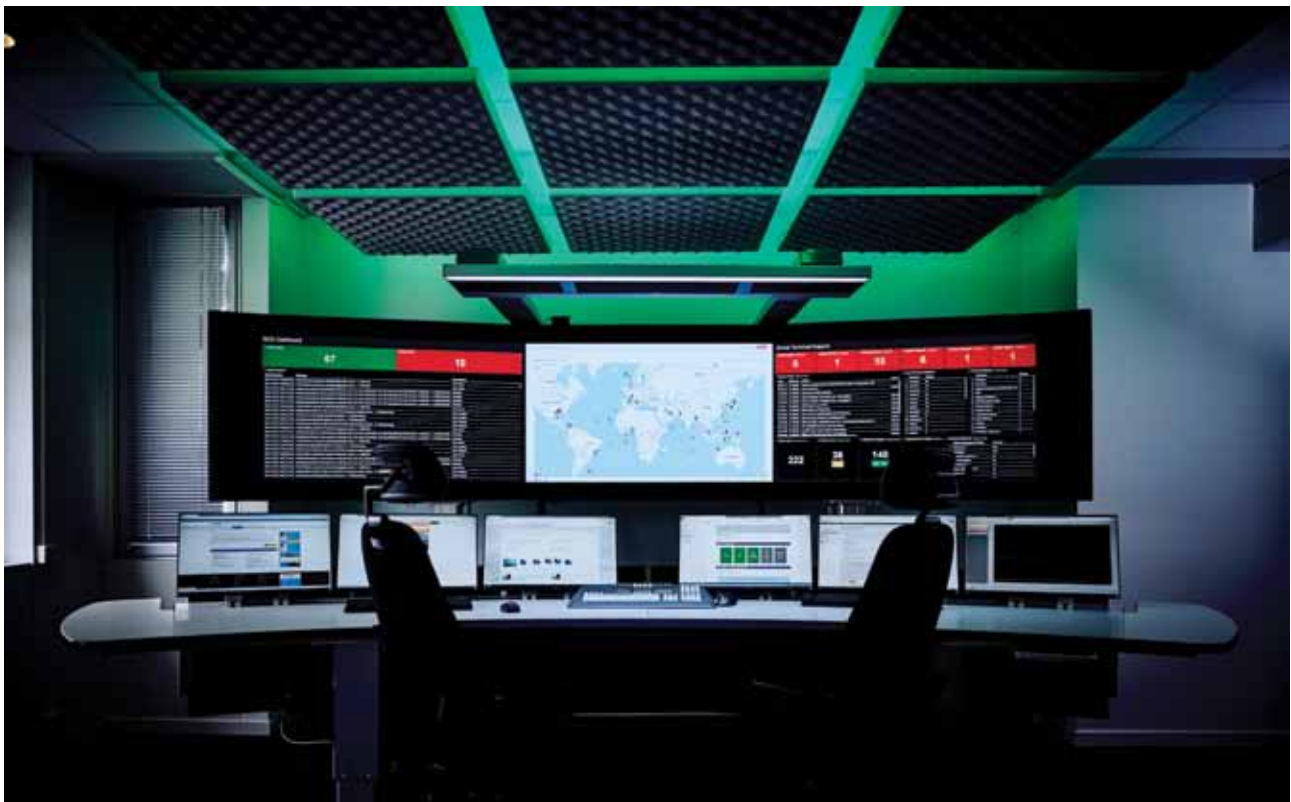
Integrated Operations Center at Billingstad
