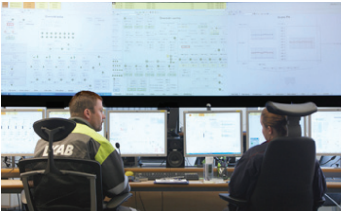
The control room with its System 800xA operator workplaces.
