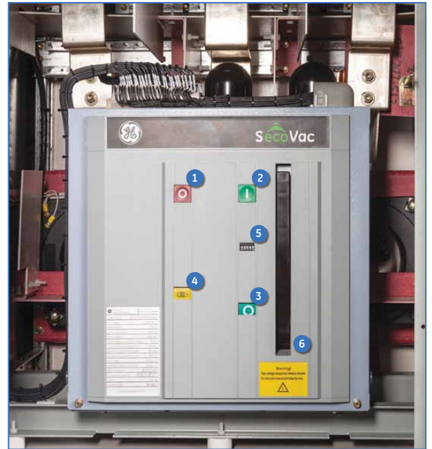
Front Panel: well-marked and easy-to-read operating controls and indicators include (1) TRIP button, (2) CLOSE button, (3) OPEN/CLOSE indicator, (4) CHARGE/DISCHARGE indicator, (5) OPERATIONS counter and (6) handle for manually charging the breaker.
