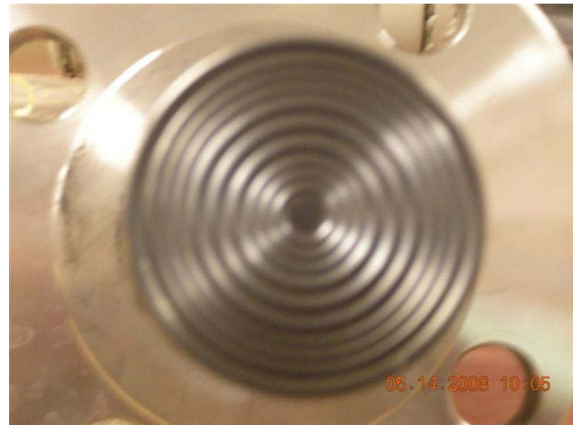
Inspection of diaphragm after eight months of service shows no adverse effects from the abrasive nature of fast flowing pulverized coal.
