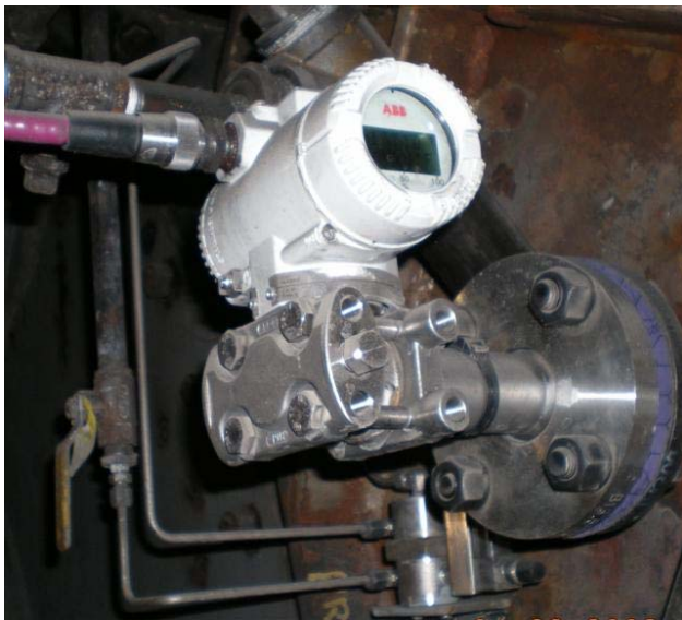
ABB 2600T pressure transmitter with direct-mount seal and Diaflex coated diaphragm. Transmitter is installed on the exhaustor of a coal pulverizing mill.
