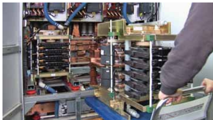
ACS 6000 phase module exchange
