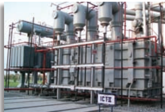
400/220/33kV Three Phase Auto Transformers
