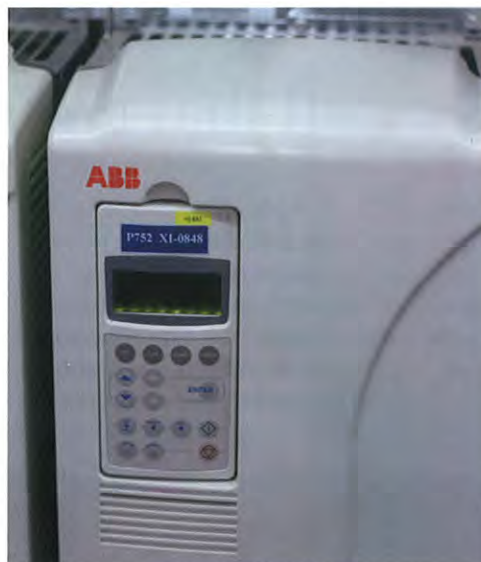
ABB Drive control at Stockstadt
