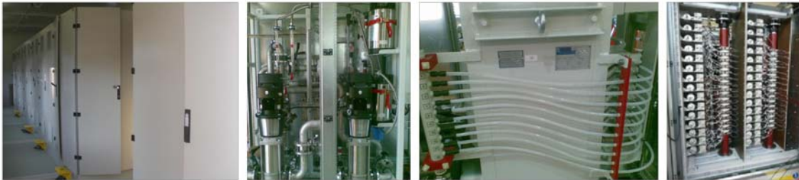
Figure 2: LCI frequency converter: overall, water cooling unit, DC link reactor, thyristor stacks
