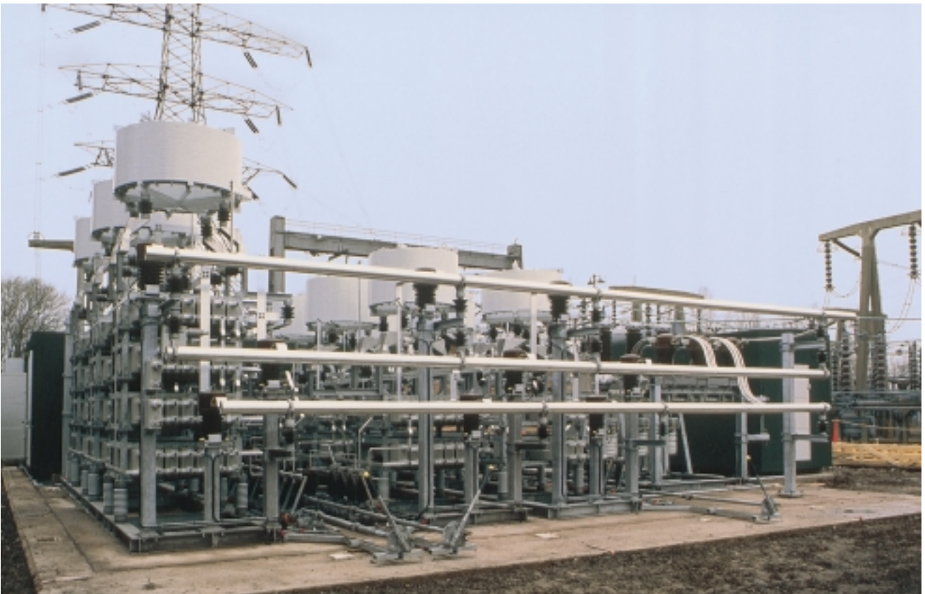
RSVC at the NGC's Penn substation
