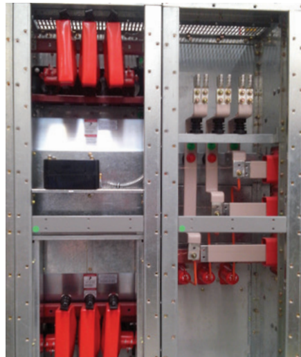
Fig. 7 Power cables compartment
