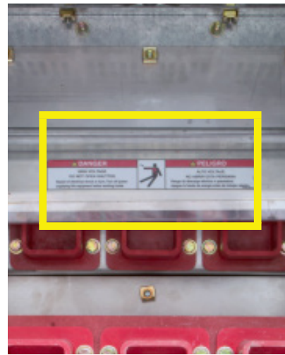
Fig. 15 Line side shutter
